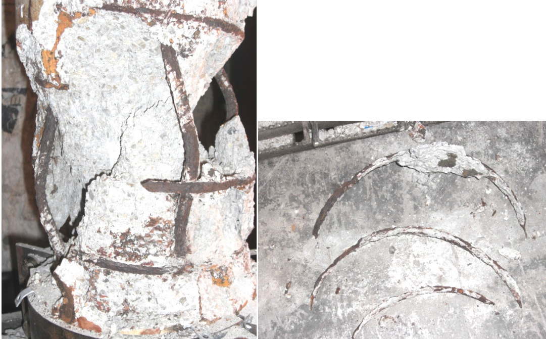
Figure 3.1: Effects of corrosion on steel spiral
