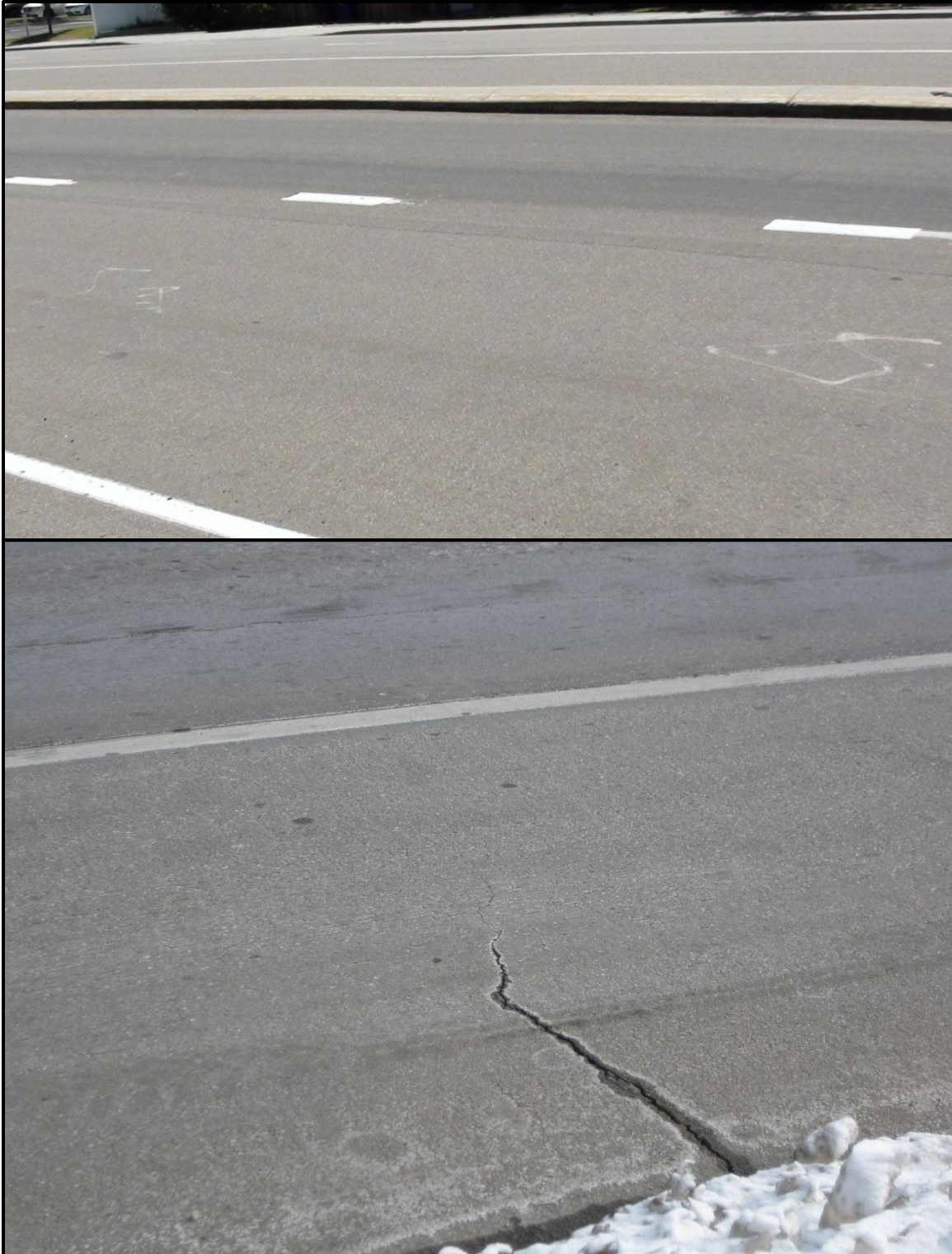
Figure 15 - SR 111 on June 13, 2012, no visible thermal distress (Top) and January 23, 2013, showing a thermal crack (Bottom)
