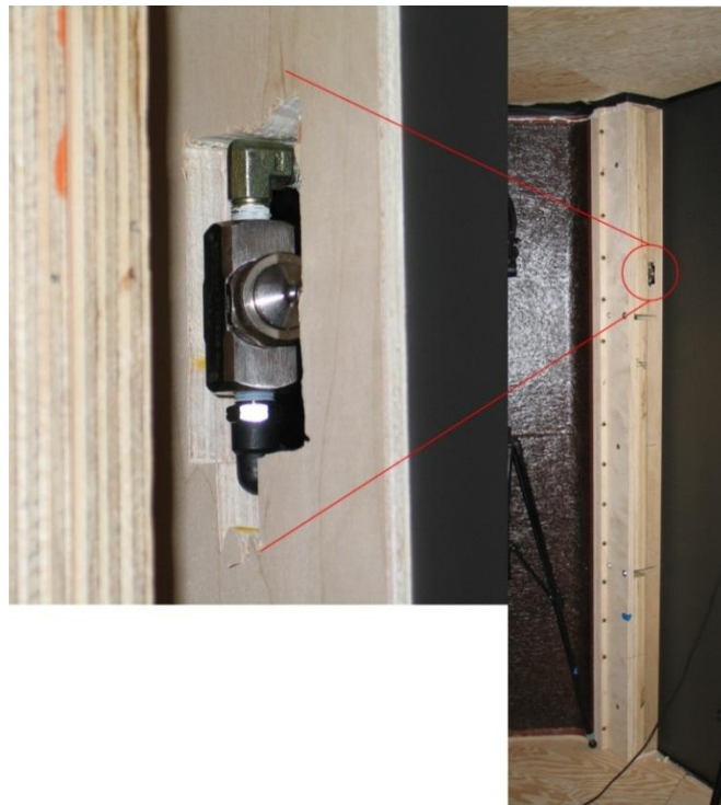
Figure 4. Nozzles position as installed with a close up of the nozzle.
