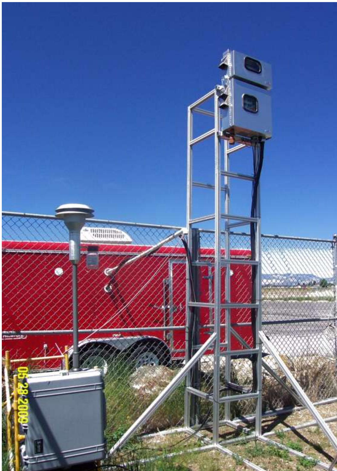
Figure 2.2. Tekran© models 1130 and 1135 mounted on a 4 m tower at the UT96 site. The Tekran© model 2537 is housed in the climate-controlled trailer.
