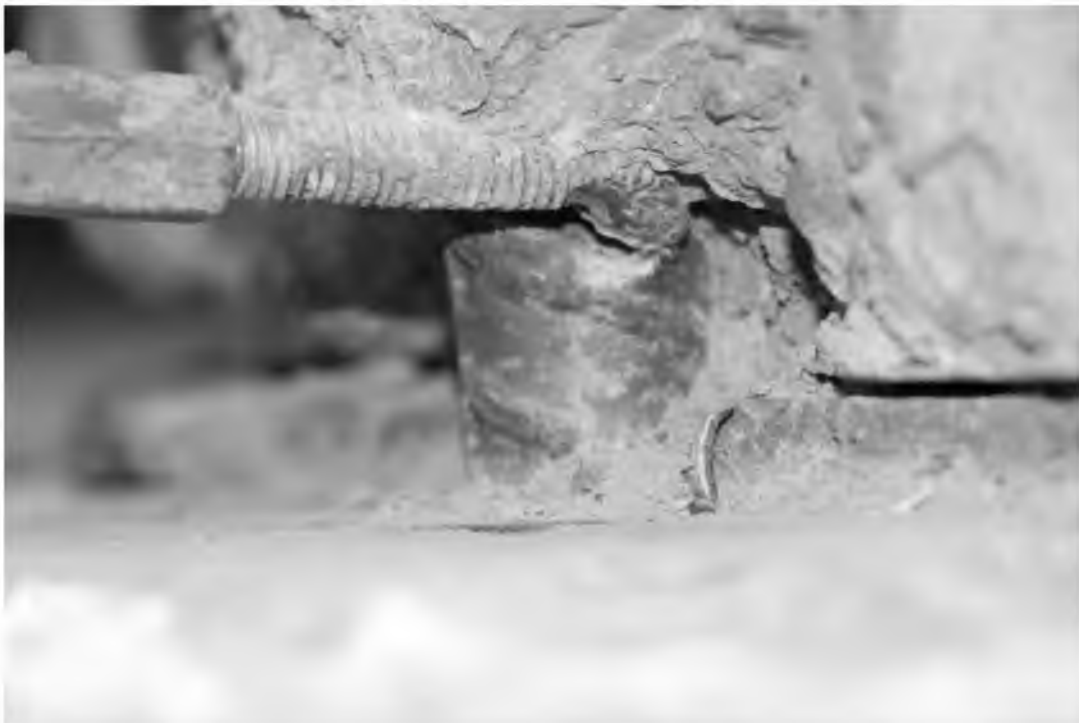
Figure 80. PCLen-2 Fractured West Longitudinal Bar
