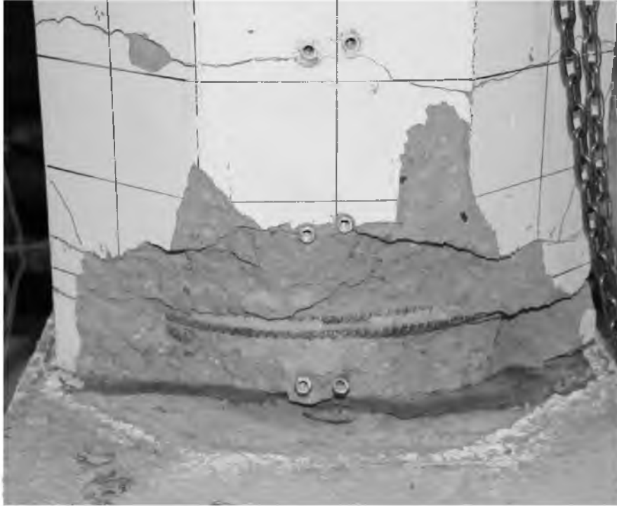
Figure 79. PCLen-2 East Face Damage
