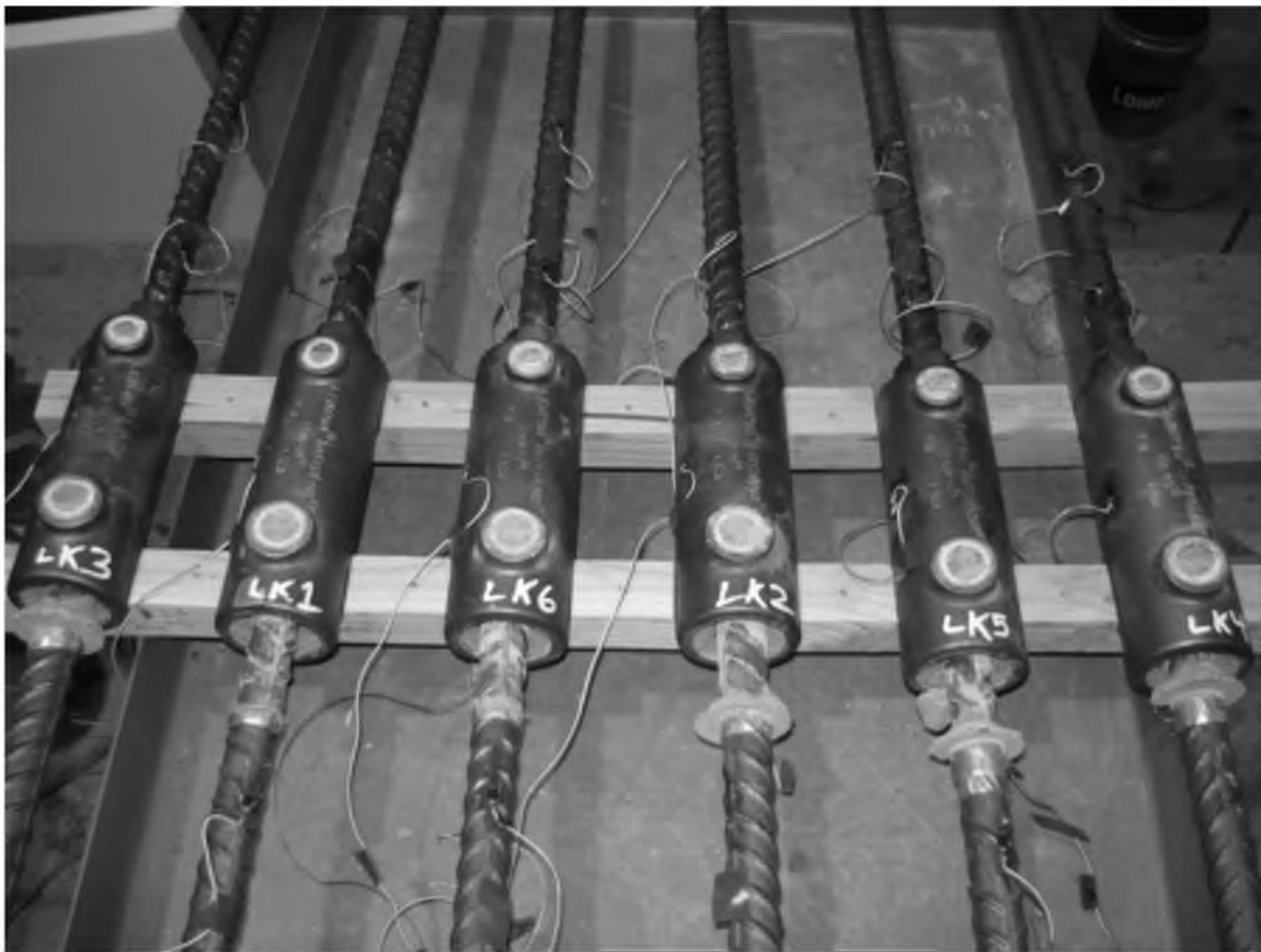
Figure 25. Lenton Interlock Splice Sleeve Failure Mode
