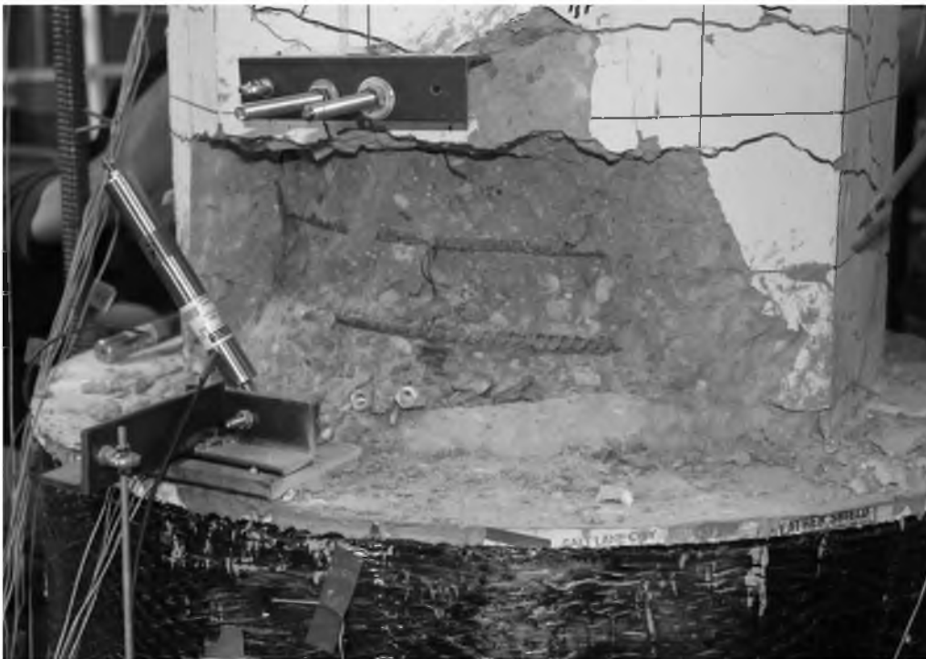
Figure 104. PCLen-2R West Face Final Damage
