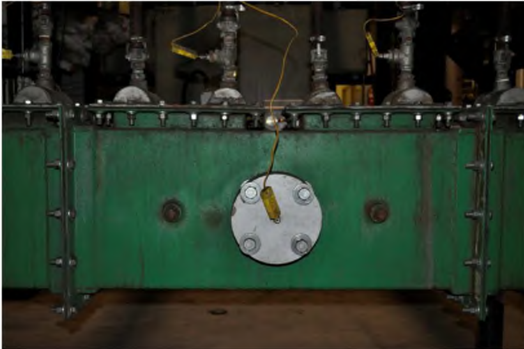
Figure 14. Heat exchanger of convective zone of OFC
