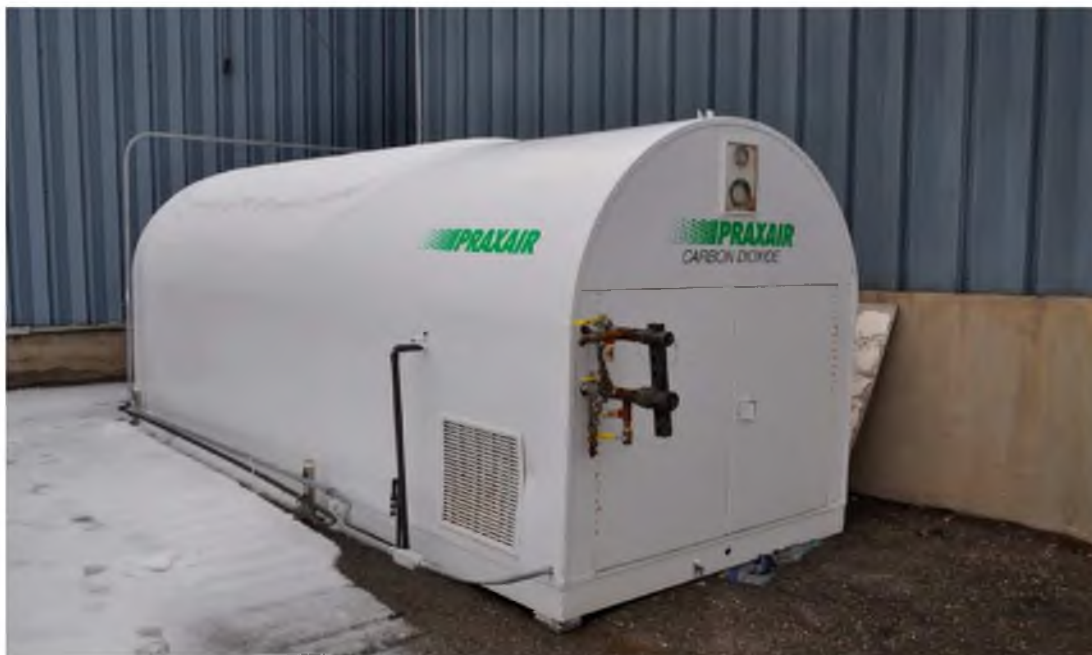
Figure 38. Carbon dioxide tank
