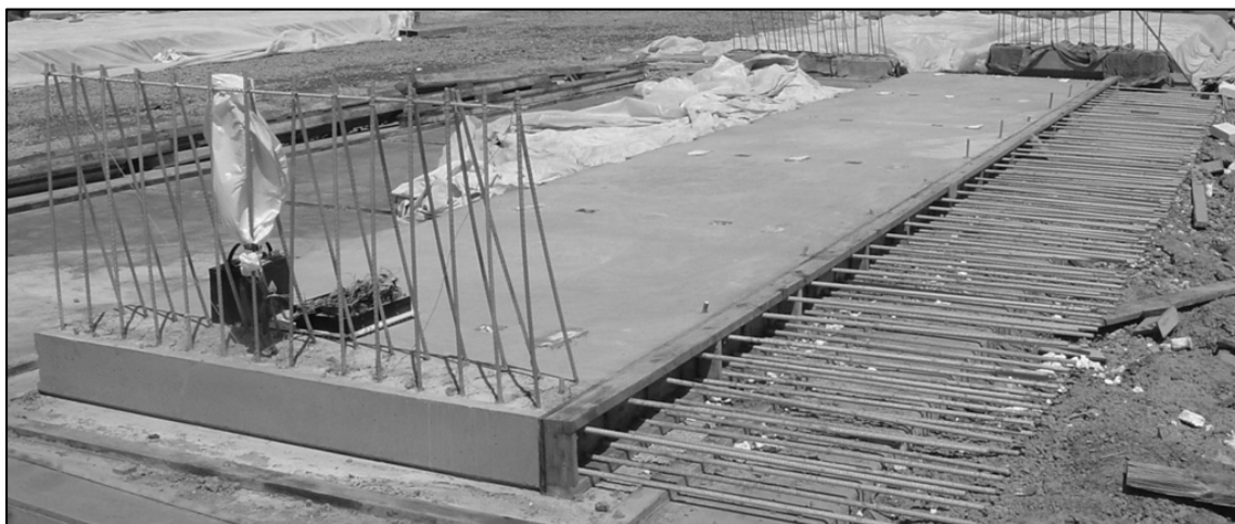
Figure 5. Panel EP3 sitting in the precast yard with approach slab rebar on the right
