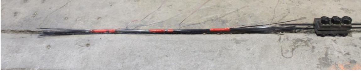
Figure 5.5: Failure of CFRP Posttensioning Rod
