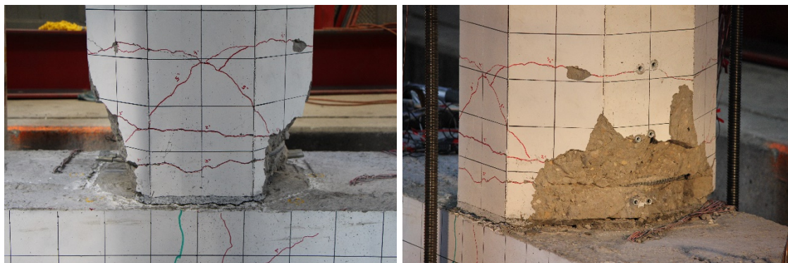
Damage state at 7% drift ratio: cracks, spalling, and exposed spiral
