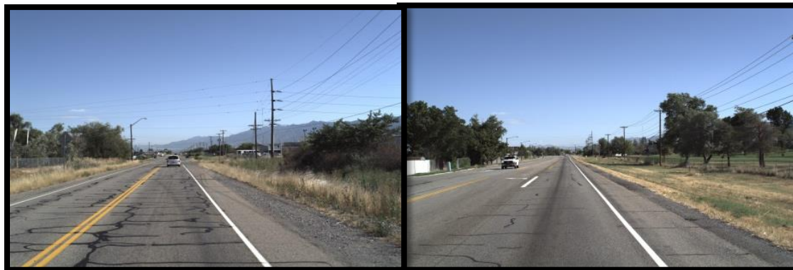
Figure 13. SR68: Raveling in the wheel path (top). Pretreatment conditions showing many tar sealed cracks (bottom).
