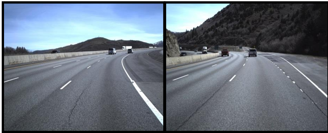
Figure 14. SR80 (3): Low severity WP cracking (left) and LNWP joint crack (right) (April 8, 2014).
