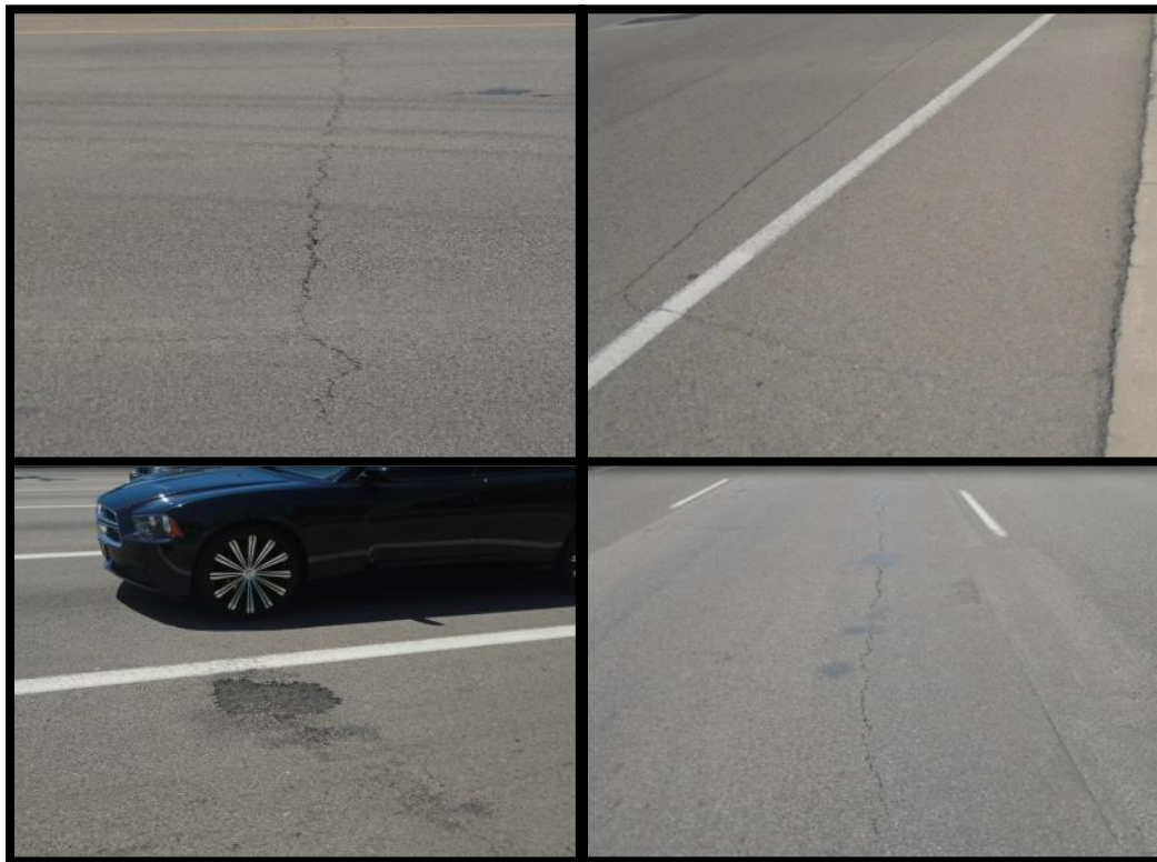
Figure 6. SR269: Top left clockwise: transverse crack, block crack, WP crack, and medium severity pothole (April 2015).
