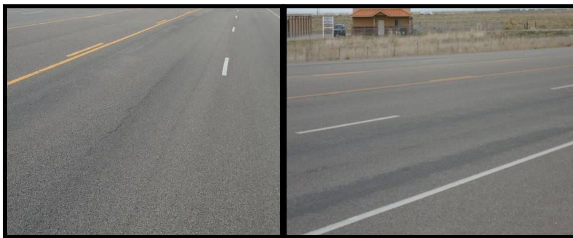
Figure 2. SR36: WP crack, possibly reflected, and typical bleeding seen in the wheel paths throughout the section (March 2015).
