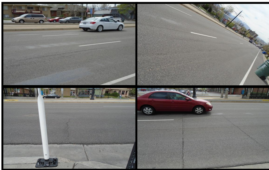
Figure 5. SR186 (2): Starting from top left to right and top to bottom: WP cracking with bleeding, additional WP cracking, transverse cracking, and block cracking (April 2015).
