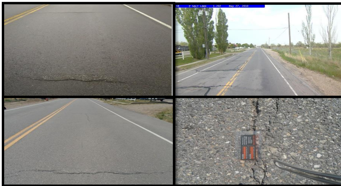
Figure 10. SR48: Transverse cracks, upper left proceeding clockwise: posttreatment (2014), pretreatment (2012), posttreatment (2015), 0.5 inch wide.
