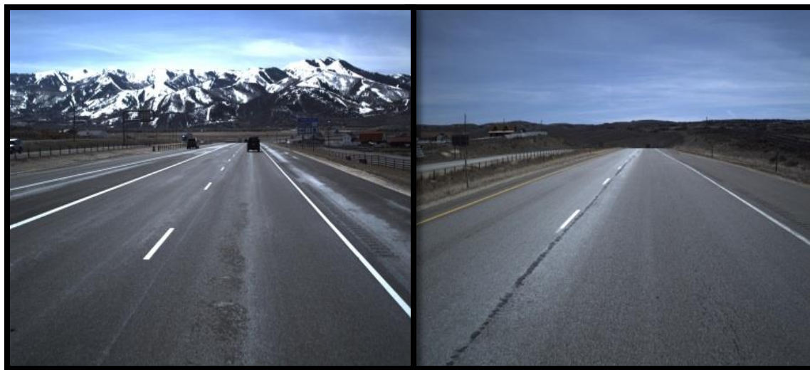
Figure 7. SR80 (1): Minor raveling and bleeding, Roadview Explorer (April 2014).
