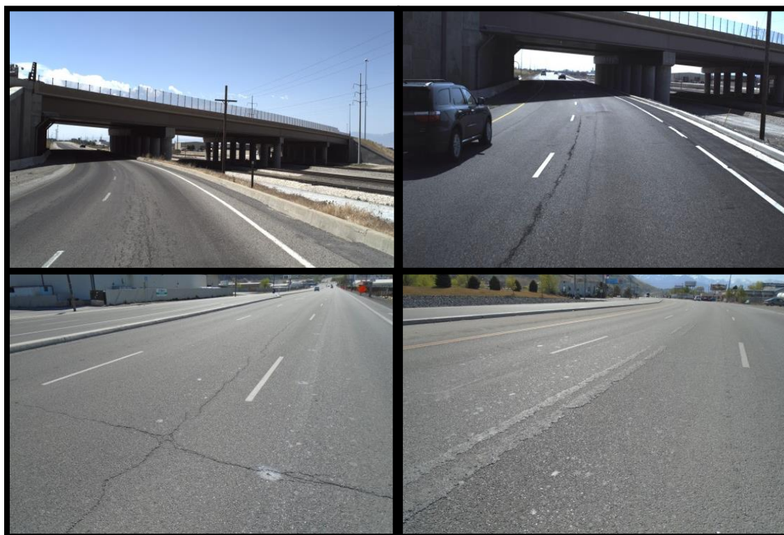
Figure 3. SR89: Top left, 2012 pretreatment fatigue damage. Top right, same location 2014. Bottom left, posttreatment transverse, and longitudinal cracking with spalling. Bottom right, medium severity bleeding (April 2015).
