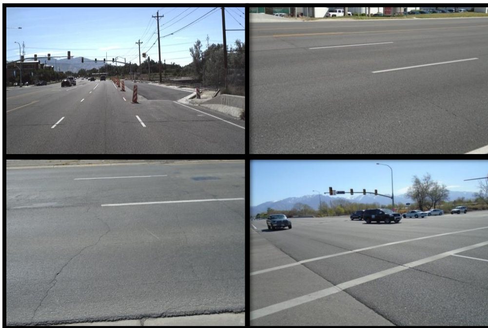
Figure 9. SR171: Top left: transverse crack posttreatment (2012). Top right: same location (2015). Bottom left: block and transverse cracking. Bottom right: LWP cracking (April 2015)
