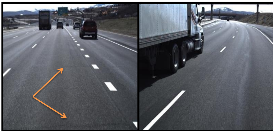
Figure 8. SR80 (2): Two minor transverse crack formations depicted on the left with minor bleeding in the center of the outside lane on the right (April 2014).
