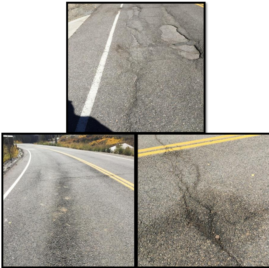
Figure 12. SR210: Delamination (top), raveling, and transverse cracking with raveling (April 2015).
