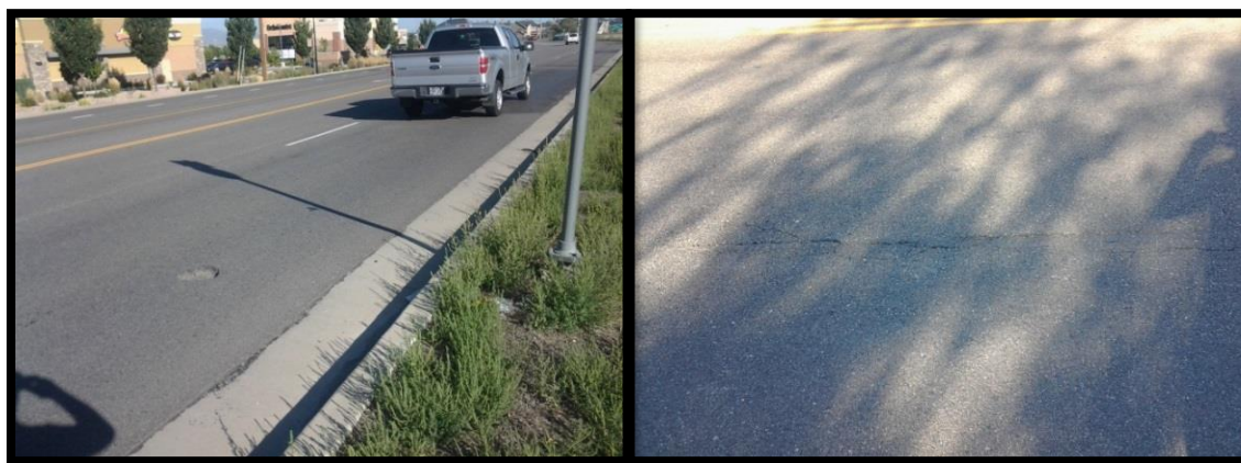
Figure 11. SR154: One of three potholes in the wheel path (left) and (right) LNWP joint crack (September 2014).
