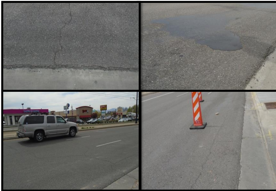
Figure 4. SR186 (1): Top left: transverse crack with raveling. Top right: medium severity bleeding. Bottom left: block cracking. Bottom right: WP cracking (April 2015).
