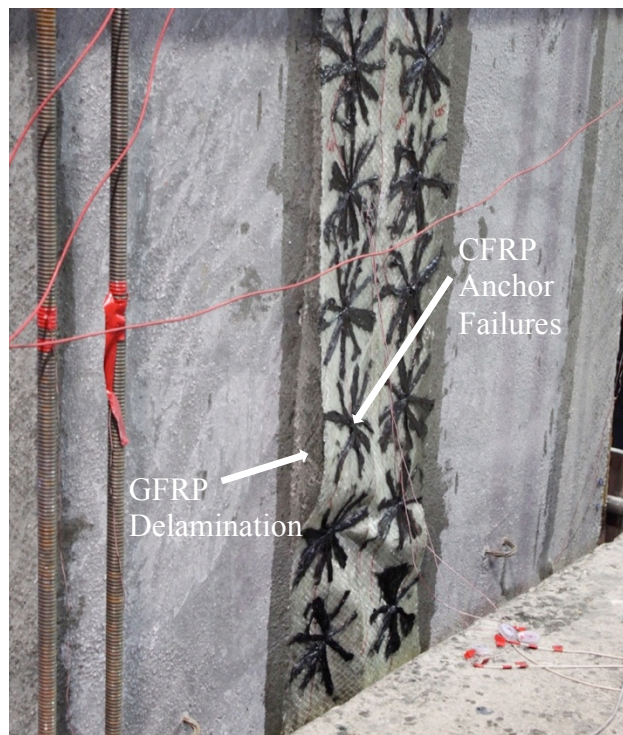
Figure 4.31 – Test #4 connection failure.
