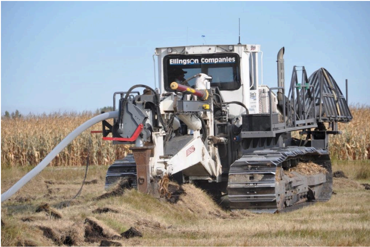
A tiling machine installed a flexible drainage tile line in a field near Fargo, ND. Photograph by Eric Brevik.
