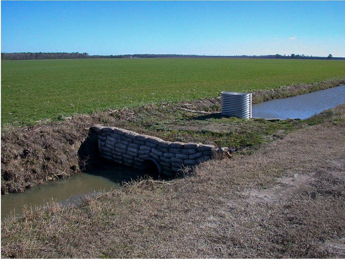
A water control structure in a North Carolina ditch. Photograph by David Lindbo.
