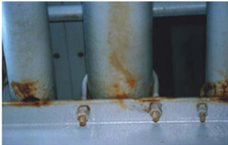
Figure 19: Another Example of Pipe Support Corrosion (Britton)
