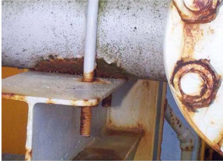
Figure 18: Example of Corrosion at Pipe Support (Young, Steve)
