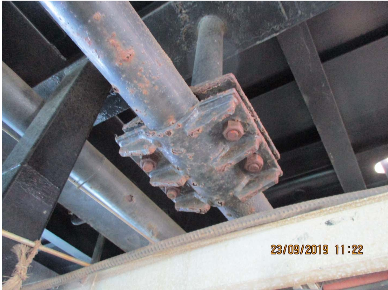
Figure 20: Another Example of Corrosion at a Pipe Support (Tillman)
