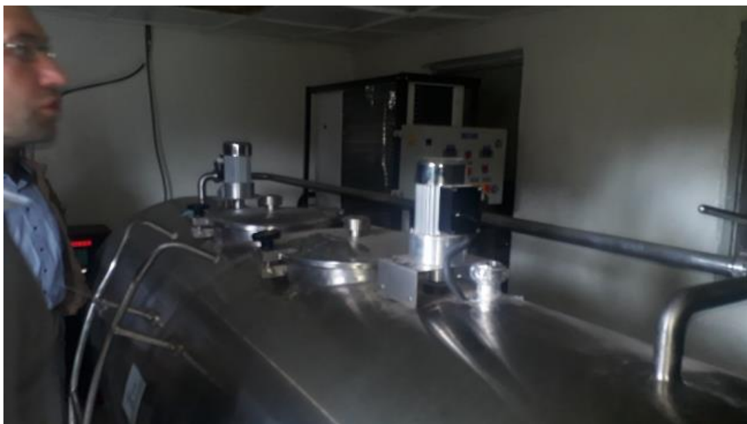
Figure 4. 2m 3 cooling tank in a chilling centre near Derba, Ethiopia. Photo: Bert Dijkink
