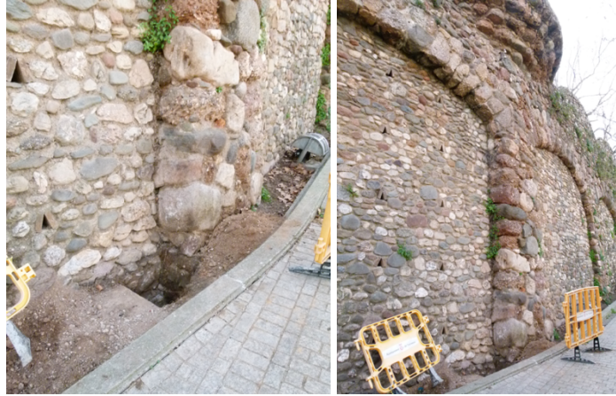
Figure A. 5. (a) Pit 7 on the left side of Buttress 5-6 (b) Location of Pit 7
