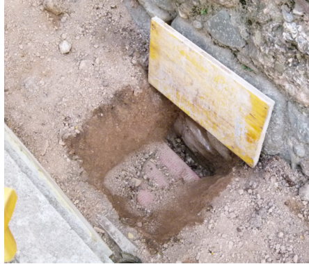
Figure A.1.Pipelines in Pit 1
