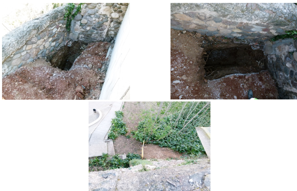
Figure A. 21. Pit 19 on the top of Buttress 9-10
