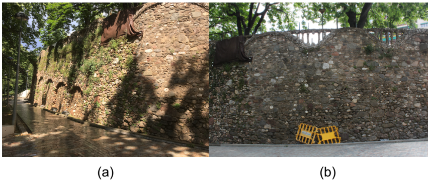
Figure 18. Mur Casa Salvans (a) Arches 1-3 located in Section 2 (b) Section 1
