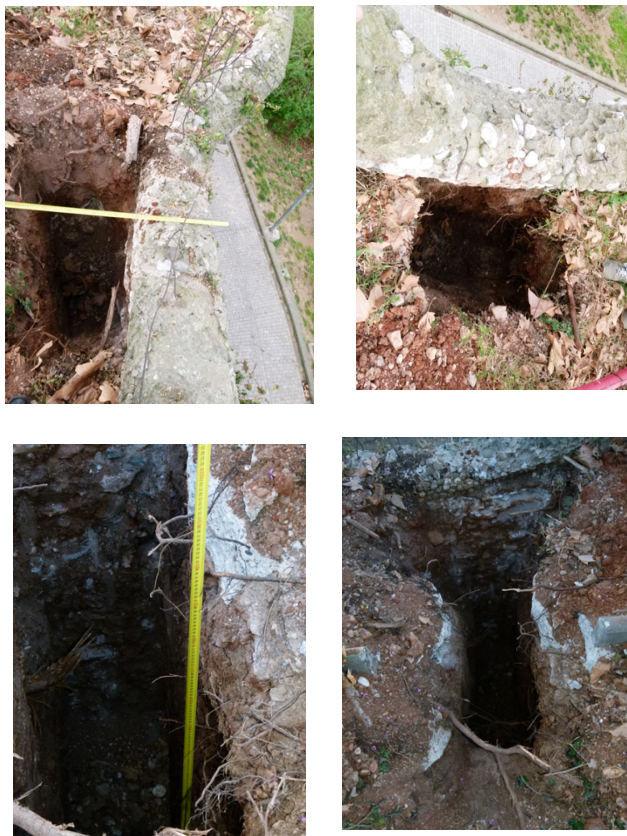
Figure A. 7. Pit 8 on the key of Arch 6 from different angles
