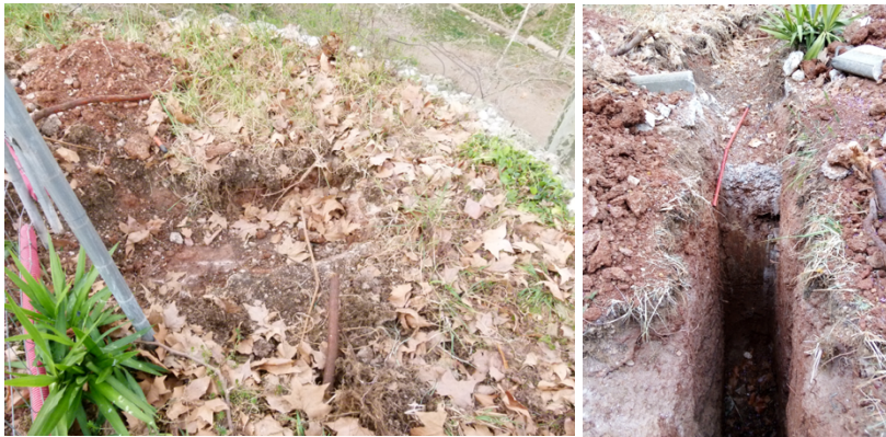
Figure A. 3(a) A Balcony section located on Buttress 5-6 from top. (b) Pit 6 on Buttress 5-6
