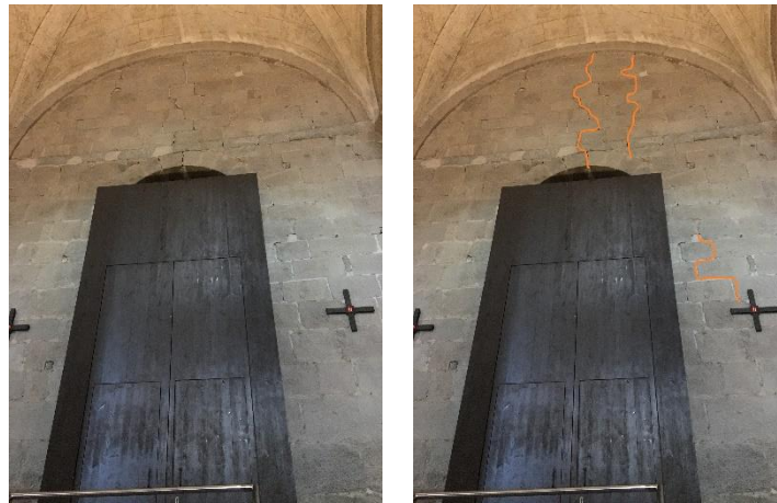
Cracks in the side walls
