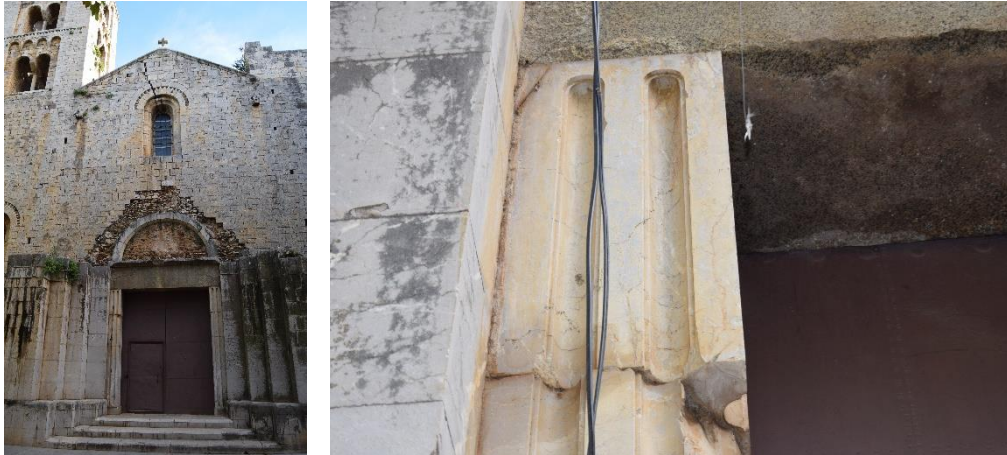
Figure 3.23. Damages in the main façade of Vilabertran
