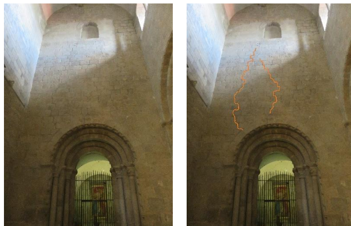
Cracks in the transept
