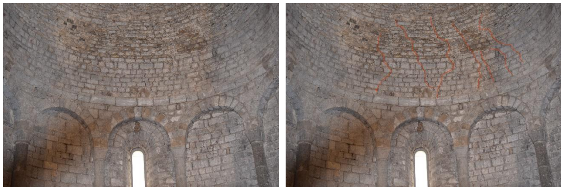
Cracks in the apse
