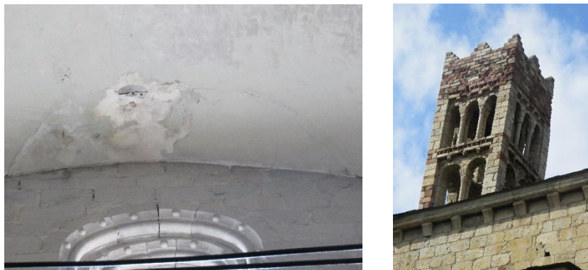
Figure 3.15. Damages due to the presence of the bell tower
