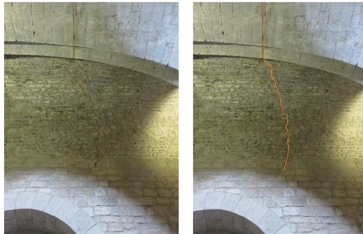
Cracks in the side wall
