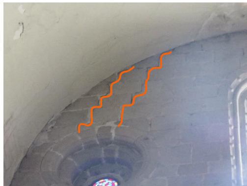
Figure 4.1. Shear cracks in the main façade of La Seu d'Ugell
