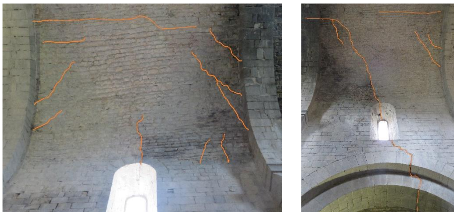
Figure 3.22. Cracks in the central vault of the nave
