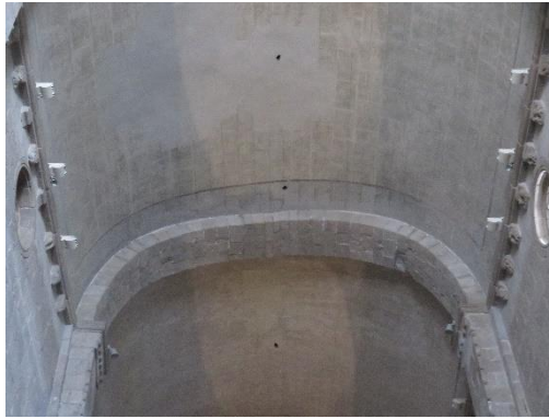
Figure 3.16. Transversal deformation of the central vault of the nave
