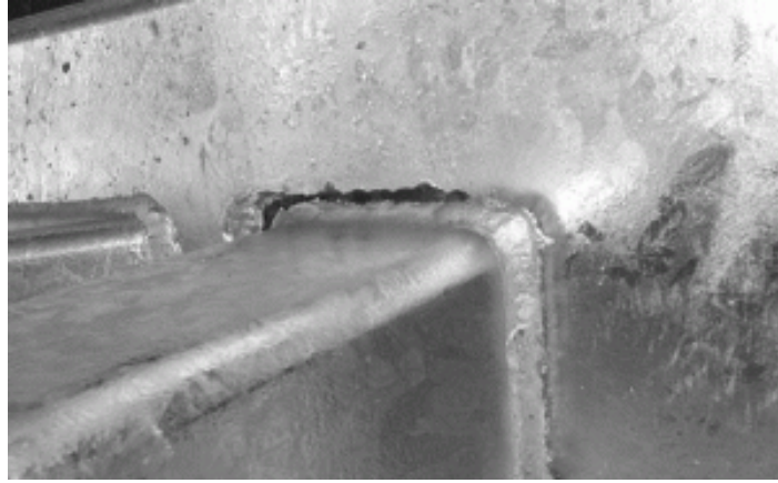
Fig. 3. Crack in heat affected zone in galvanized coating [26].
