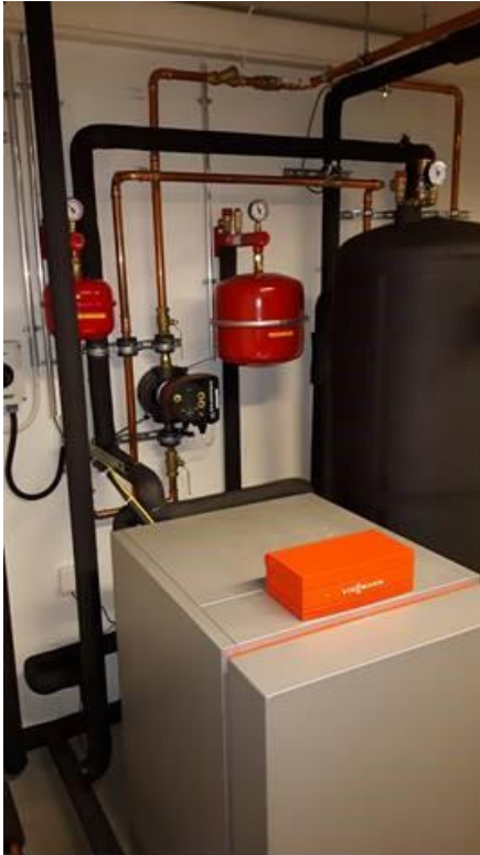
Vitocal 300-G heat pump, buffer tank and view to main piping
