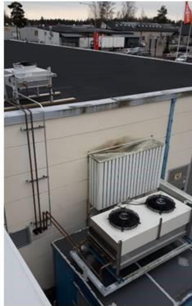
Dry cooler and heat exchanger for CO2 system
