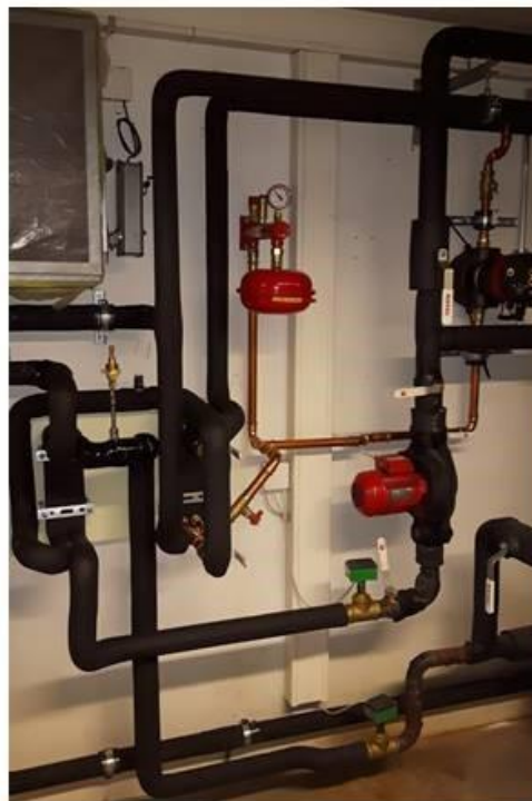
Heat exchangers and associated piping
