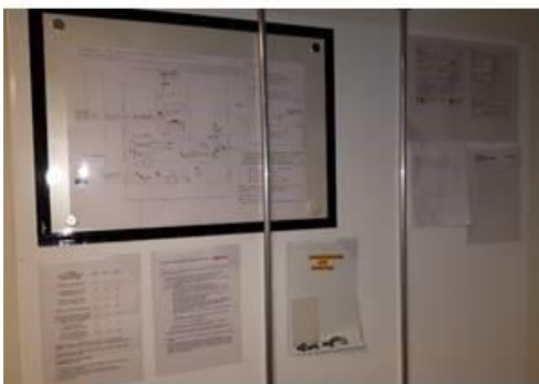
Refrigeration plant's information board
