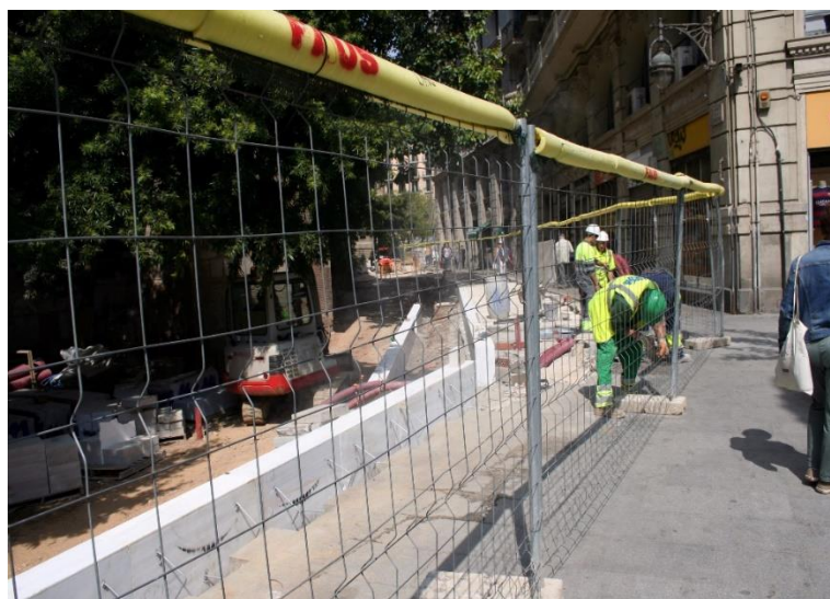
Fig.6.13. Laborers working on the construction of a “podium” to enhance the Roman Walls of Barcelona, street Tapineria, on May 2016. Ana Pastor.
