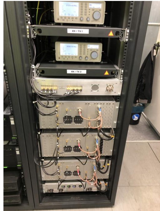
Fig. 7. RF rack. From top to bottom: redundant transceivers, switching matrix, VHF/UHF/S Band frontends, PSU
