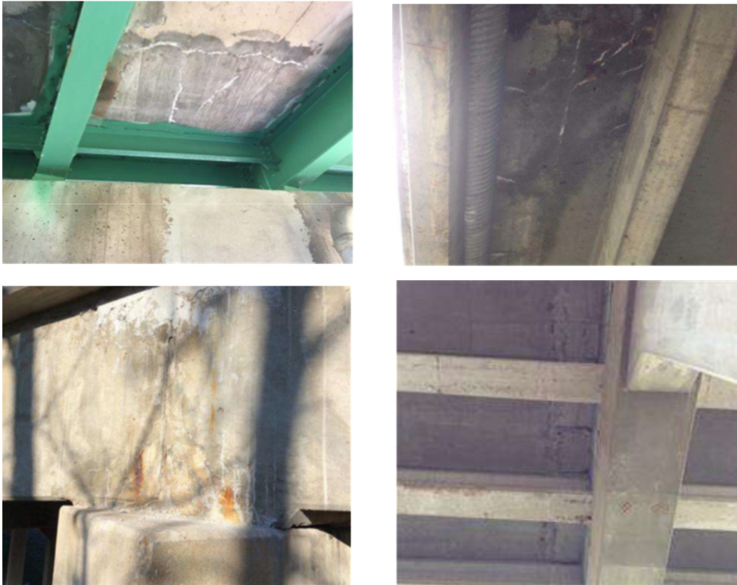
Figure 2.18: Cracking in Indiana link slab bridges as reported in inspection reports
