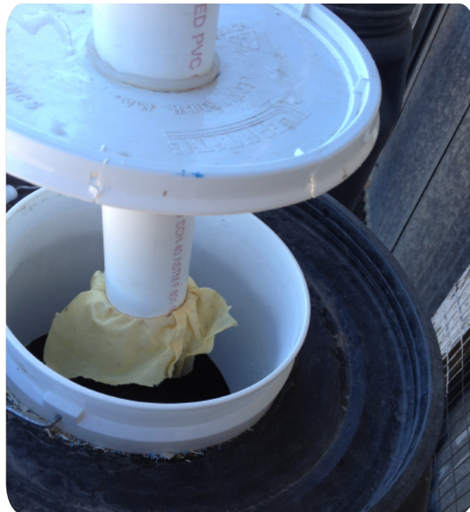
Gutter downspout with cloth screen to catch debris before entering the water storage container.
