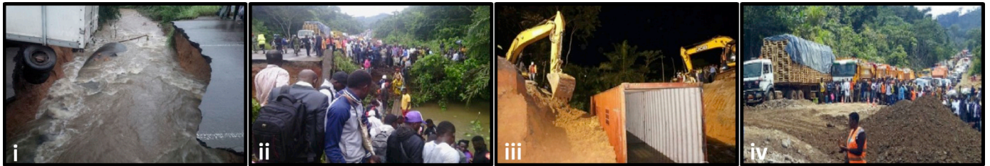
Fig. 5. (i) Collapse bridge at Manyai (ii) Stranded passengers at collapse bridge (iii) Quick fix of collapsed bridge using a container (iv) Queue of vehicles waiting for the bridge to be fixed. Source: Various- [47,48].
