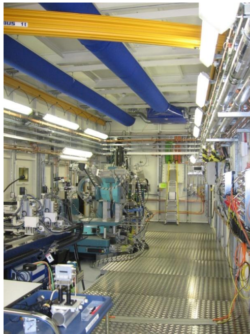
Figure 23 - B16 Hutch showing air distribution socks
