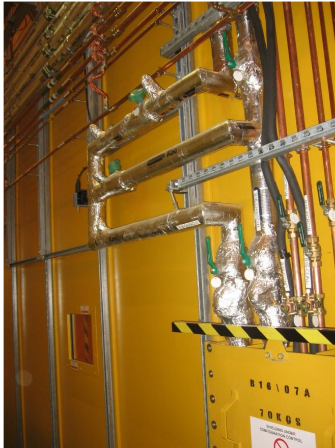
Figure 24 – Location of 3 port valve outside the hutch
