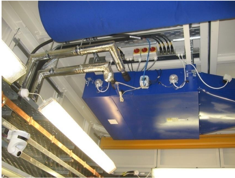
Figure 22 – Hutch roof mounted air chiller and fan
