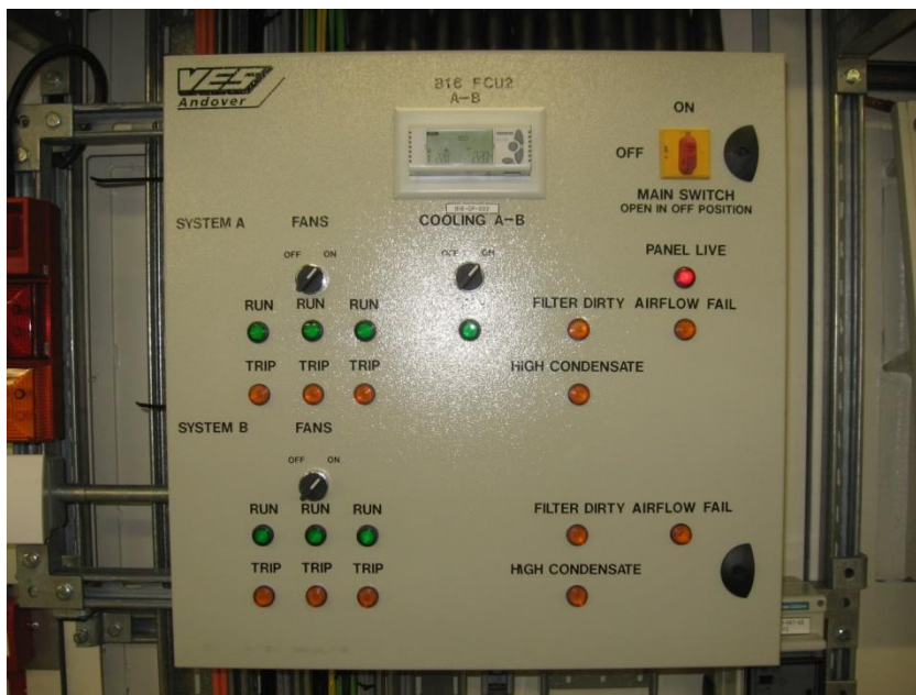
Figure 26 – Air temperature control panel
