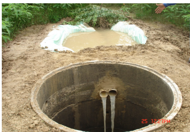
Fig. 50 Rainwater recharge to dilute groundwater
