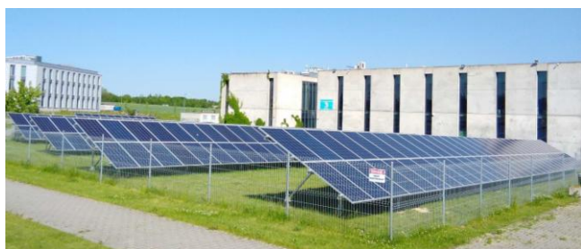
Fig. 2. Photovoltaic plant in front of the building of the Lublin Science and Technology Park [33]
