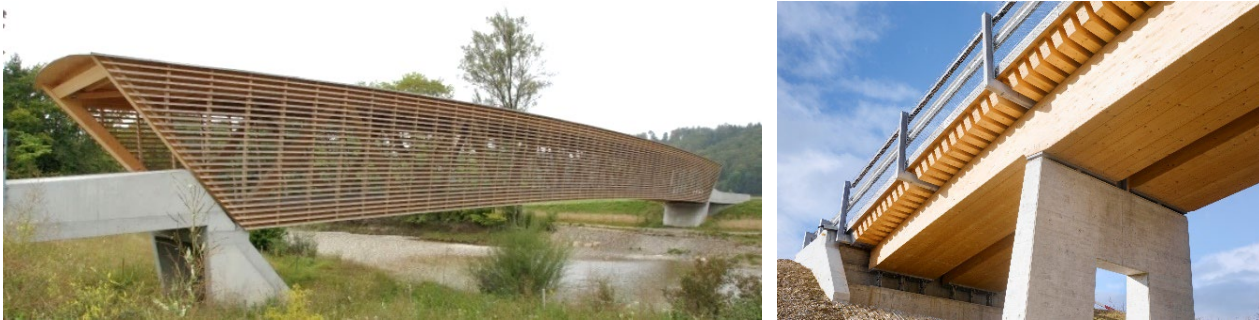
Figure 39: Bridge Neumatt with protected truss system using gladding (left) and Bridge Horen with weather protection by structural overhang
