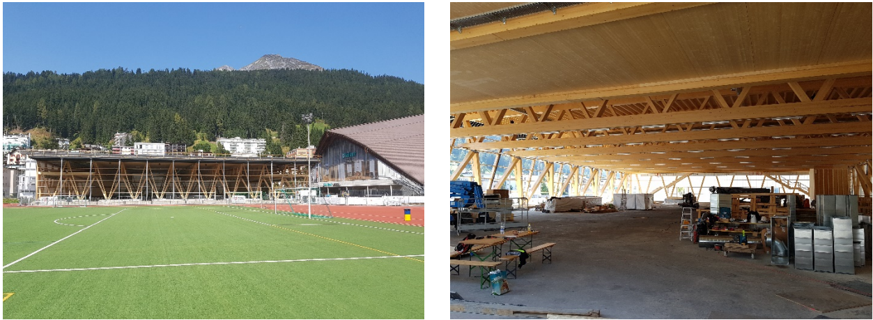
Figure 22: View of the outside and inside of the ice rink during construction
