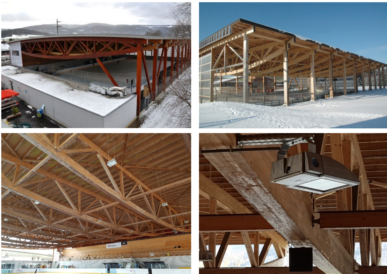
Figure 19: Pictures of the outside and inside of the ice rinks of Delémont (upper left) and Le Locle (upper right) (sources unknown) and pictures of the interiors of the Delémont ice rink with the ice formation on the downward facing surfaces of the load bearing members (bottom right)
