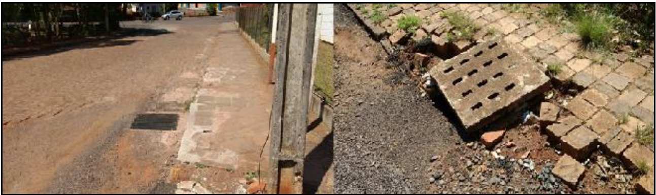
Figure 2 – Photographic records at the first flooding point
