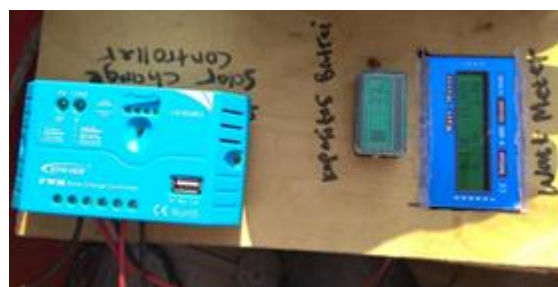
Fig 7. Solar charge controller
