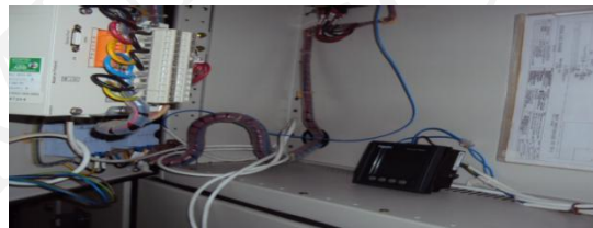
Figure 7: PowerLogic Power Meter
