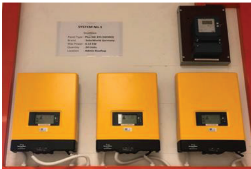
Fig. 2. Installation of 6kW Inverters for monocrystalline PV system at PVSG Lab Weather Station, UTeM
