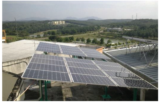
Fig. 3. Monocrystalline PV module at roof top of FKE, UTeM
