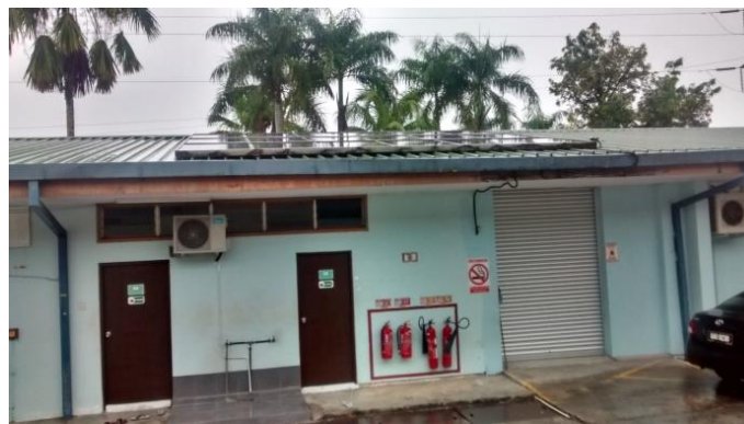
Figure 3: Solar panels installed on the roof of the LEA
