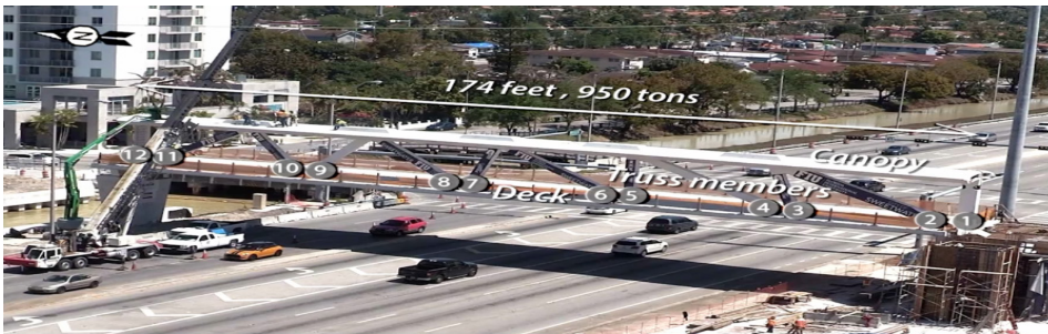
Fig. 1. Main span of the bridge before collapse.
