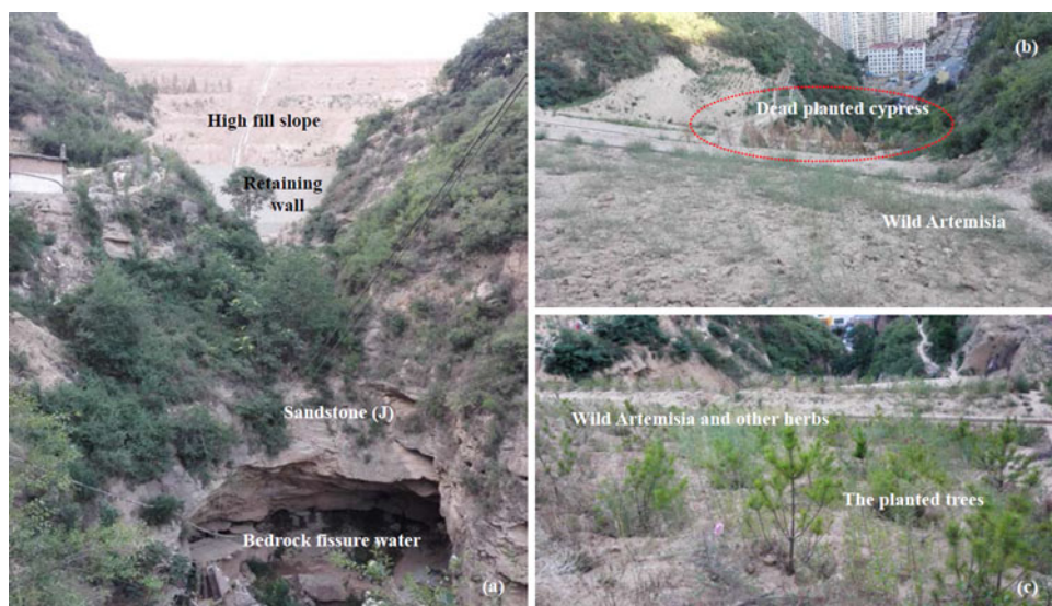
Figure 14. Huangjiaguagou high fill slope. a) An overview of the slope (July 2015), b) the growth state of plants (July 2015) and c) the growth state of plants (July 2016).
