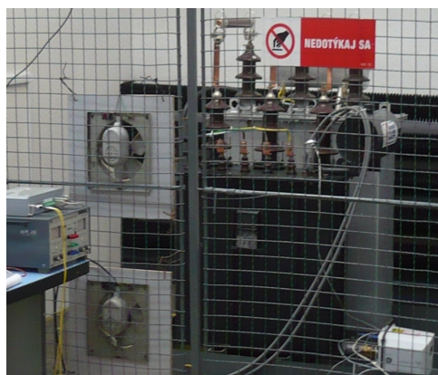
Fig. 8. View of the measured transformer and the NEOPTIX T system
