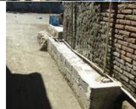
Figure 3. Disposal system in non-stage housing units
