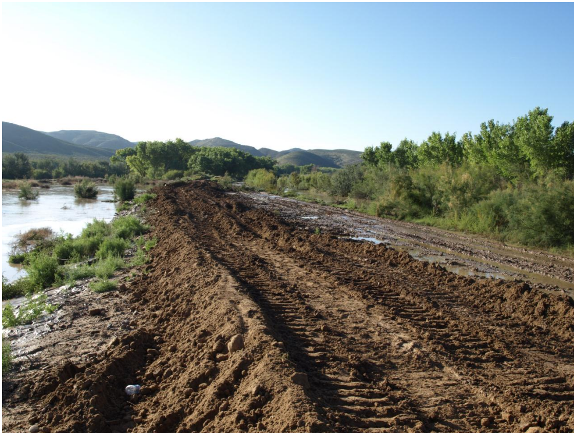
Photo 8: Temporary fix of spoil levee between Drain Unit 7 Extension and the Rio Grande (September 2013, AuBuchon)
