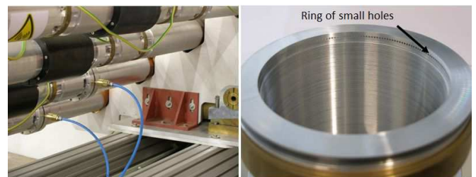
Fig. 5. Waveguide ventilation system. Dry air supply mounted on waveguide flanges (left), ring of cutoff holes at the end of a corrugated waveguide (right).
