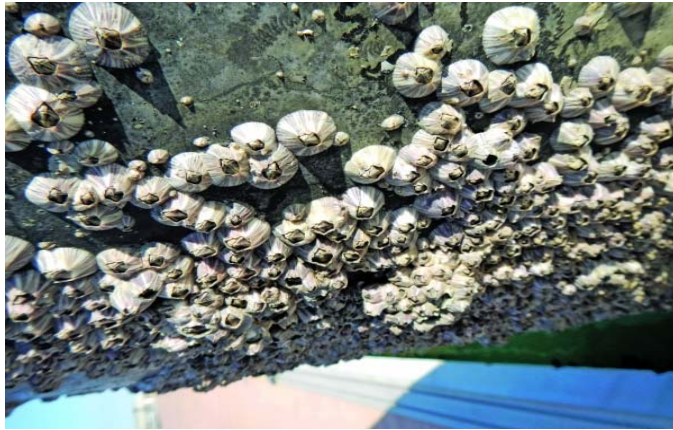
Figure 6 Shell fouling accumulation
