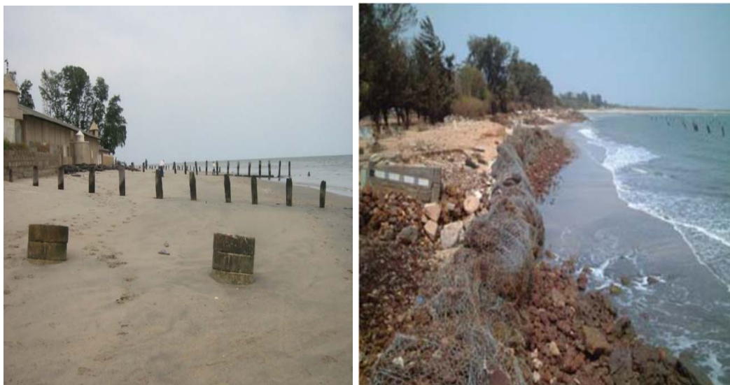
Figure 13: Palm groynes & gabion baskets as sea defence measures in Banjul
