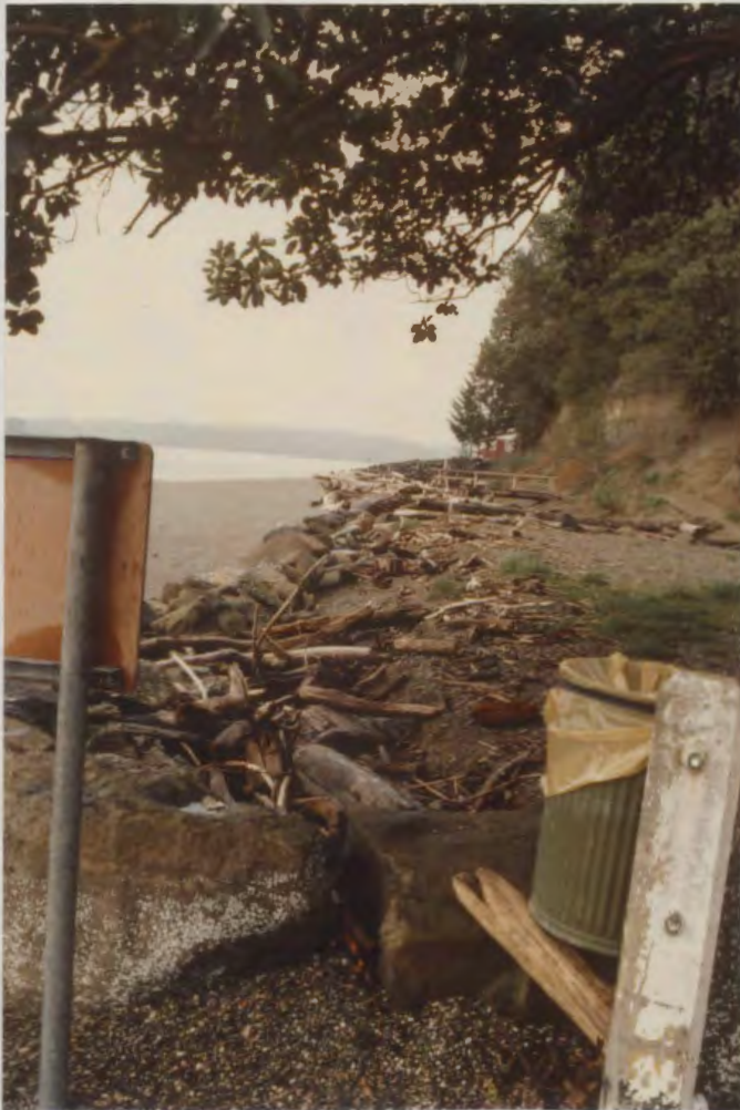
FIGURE 18b. View north showing the erosion of fill emplaced the previous year after one winter storm season. Photo taken 3/30/83.
