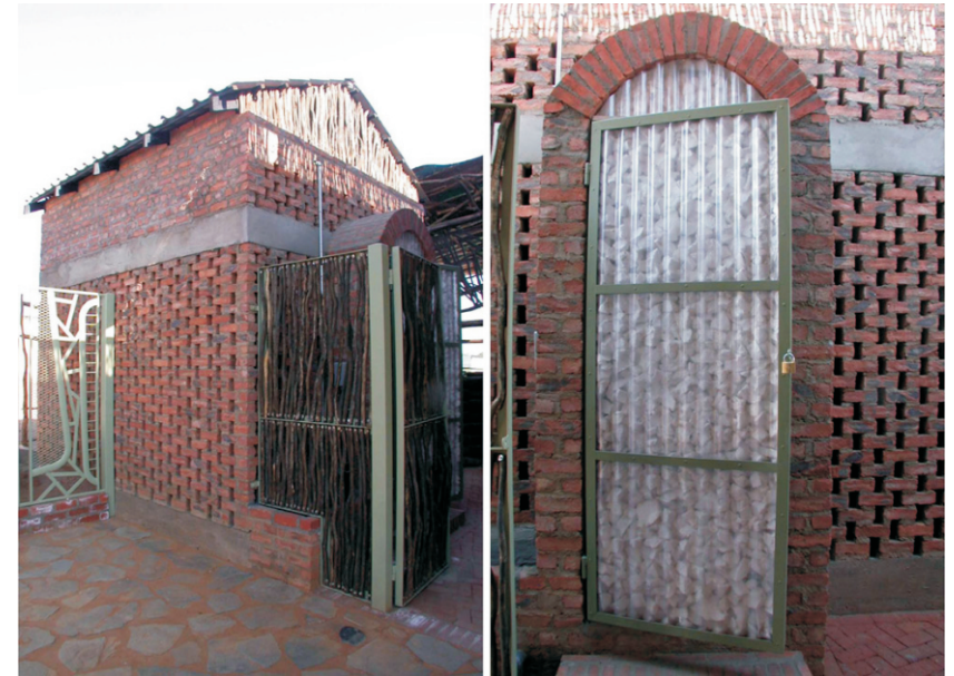
Figure 082. Sustainable practices, like filling the cooling tower door with foam as insulation provides opportunities for education.
