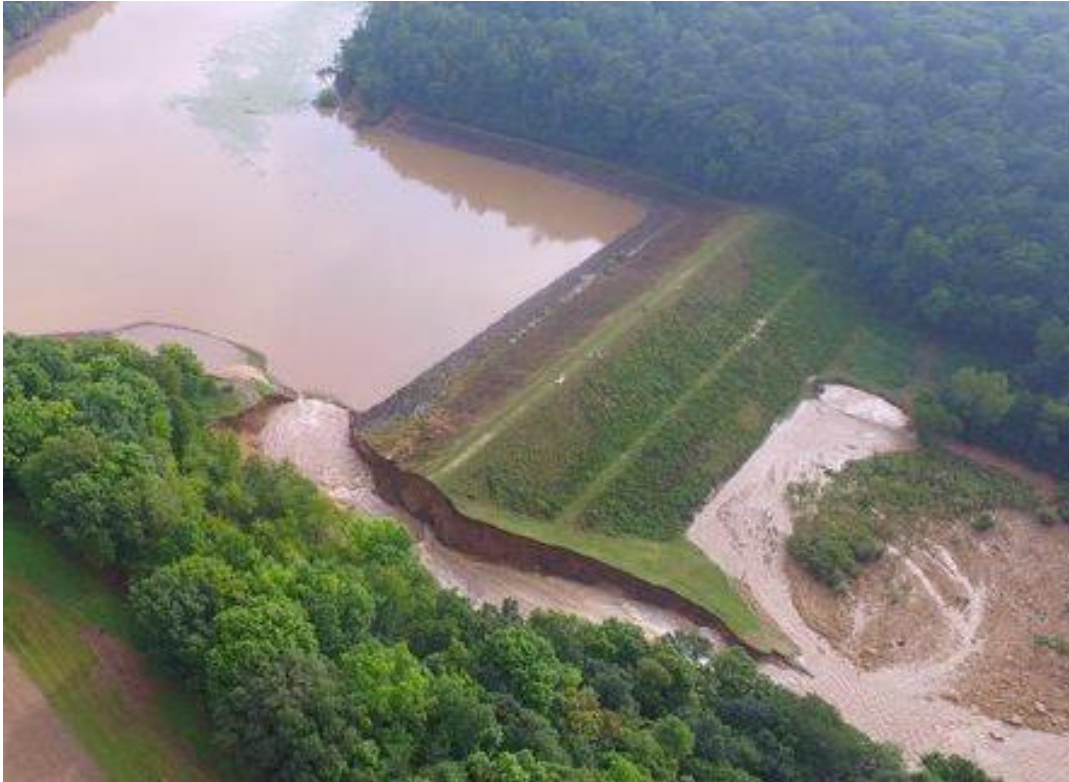
Figure 1- Jersey Valley dam breach, August 2018
