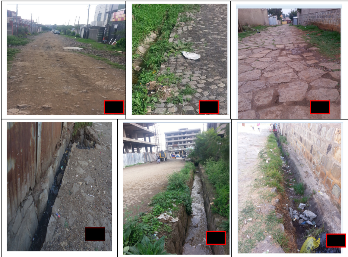
Fig. 3. Common road pavements, in addition to asphalt: Gravel (A) ( 8^{\circ}59'19.901''\text{N} & 38^{\circ}43'33.453''\text{E} ), Cobblestone (B) ( 8^{\circ}59'9.81''\text{N} & 38^{\circ}43'51.904''\text{E} ), and stone paver (C) ( 9^{\circ}3'0.519''\text{N} & 38^{\circ}44'33.77''\text{E} ) and drain types along Gravel (D) ( 9^{\circ}2'58.893''\text{N} and 38^{\circ}44'37.087''\text{E} ), Cobblestone (E) ( 8^{\circ}58'57.67''\text{N} and 38^{\circ}43'54.859''\text{E} ) and stone paver roads (F) ( 9^{\circ}3'4.414''\text{N} and 38^{\circ}44'52.087''\text{E} ) in the case studies.
