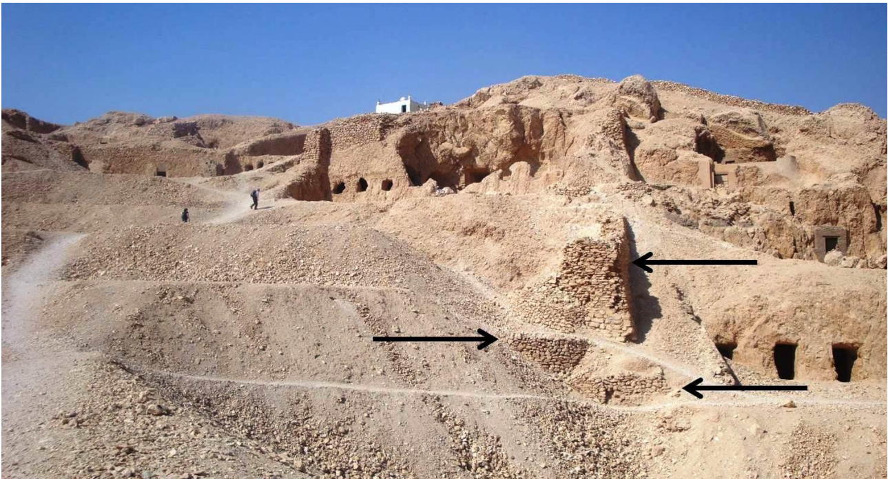
Image 17 - The northern retaining wall of the artificially constructed courtyard of TT 71. Notice the thickness at the base indicated with arrows. Photograph by Hanne Siegmeier, 2011.
