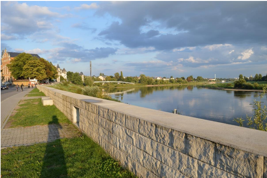
Figure 32. Floodwall in Pieschen , western part of Dresden. Low wall solution, where steel plate extensions can be fitted on top. Photo: Kristoffer Albris, July 2014.
