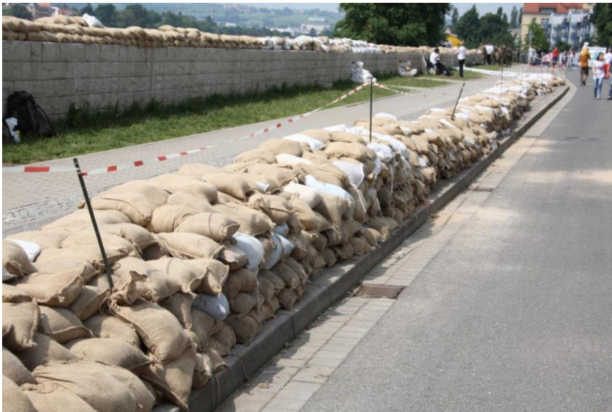
Figure 20. Wrongly placed sandbags along Kötzschenbroder Strasse in Dresden. Bags have been placed on top of the permanent floodwall, which prevents the fixing of a steel plated extension on top of the wall. Sandbags behind the wall would be overflowed in minutes if the water overtopped the wall. Photo by the Dresden Fire Department (Friedrich 2013), June 2013.
