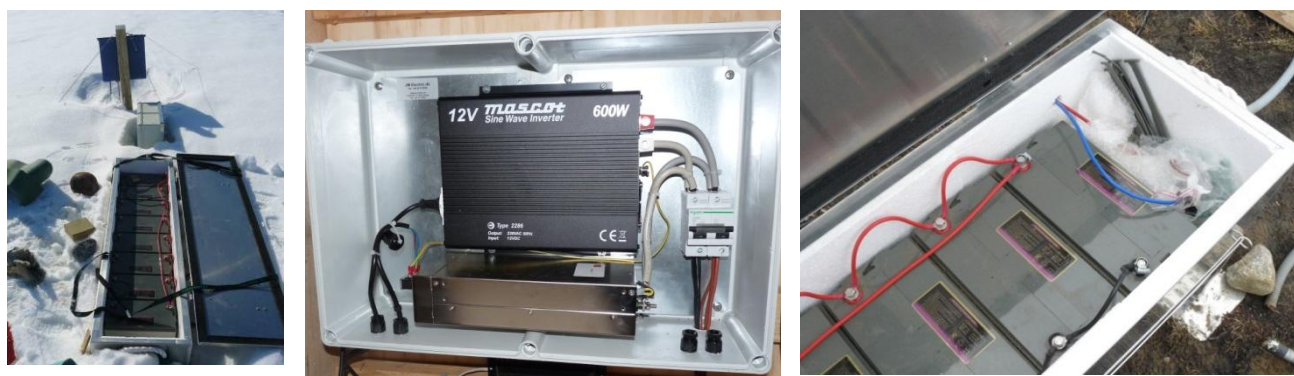
Fig 10.15 The battery box (left). A look into the transformer box, inside the hut (mid). Power cable from the instrument box enters the battery box in the southern end –the red and blue cable are connected to plus and minus on the last battery in the row.
