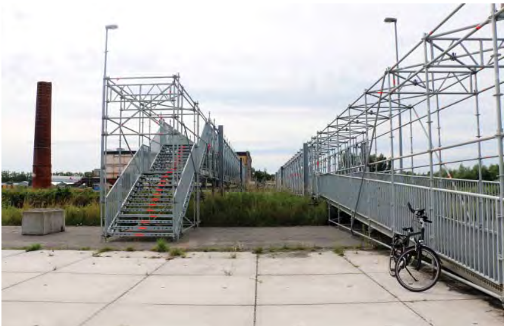
⌘ 12.08.2015_The gate in front of the scaffolding bridge –Today it is open
