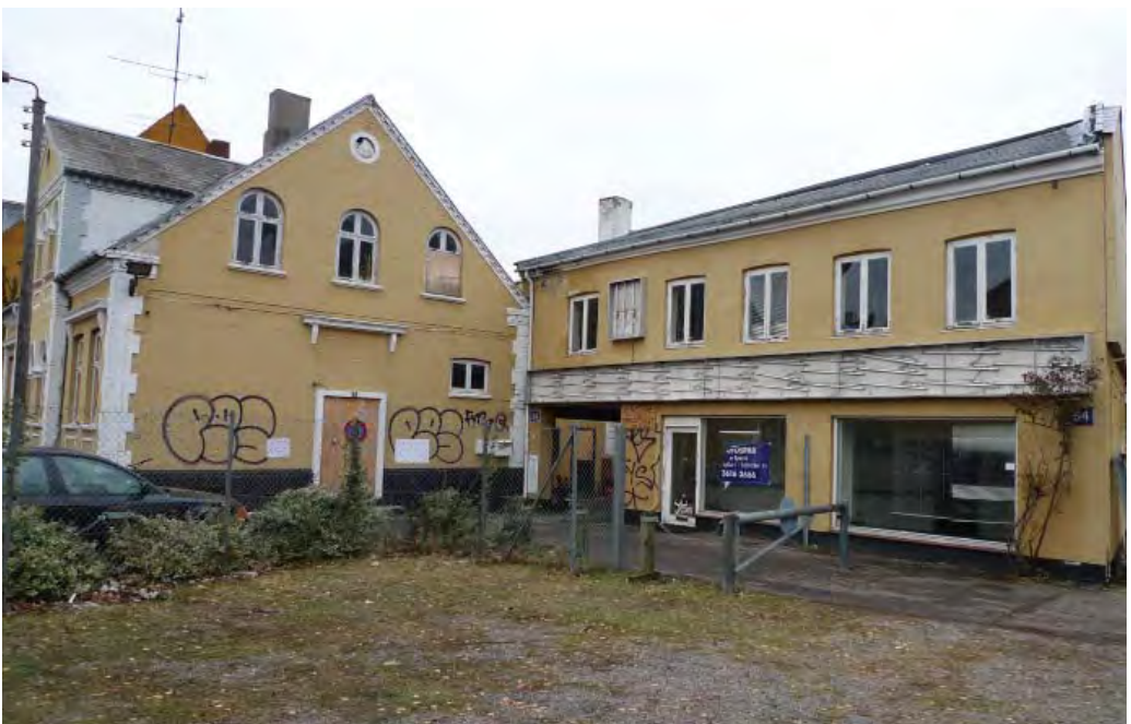
20.12.2012_ To the left the former residential building which has been defined as worthy of preservation and to the right the former car dealer shop.
