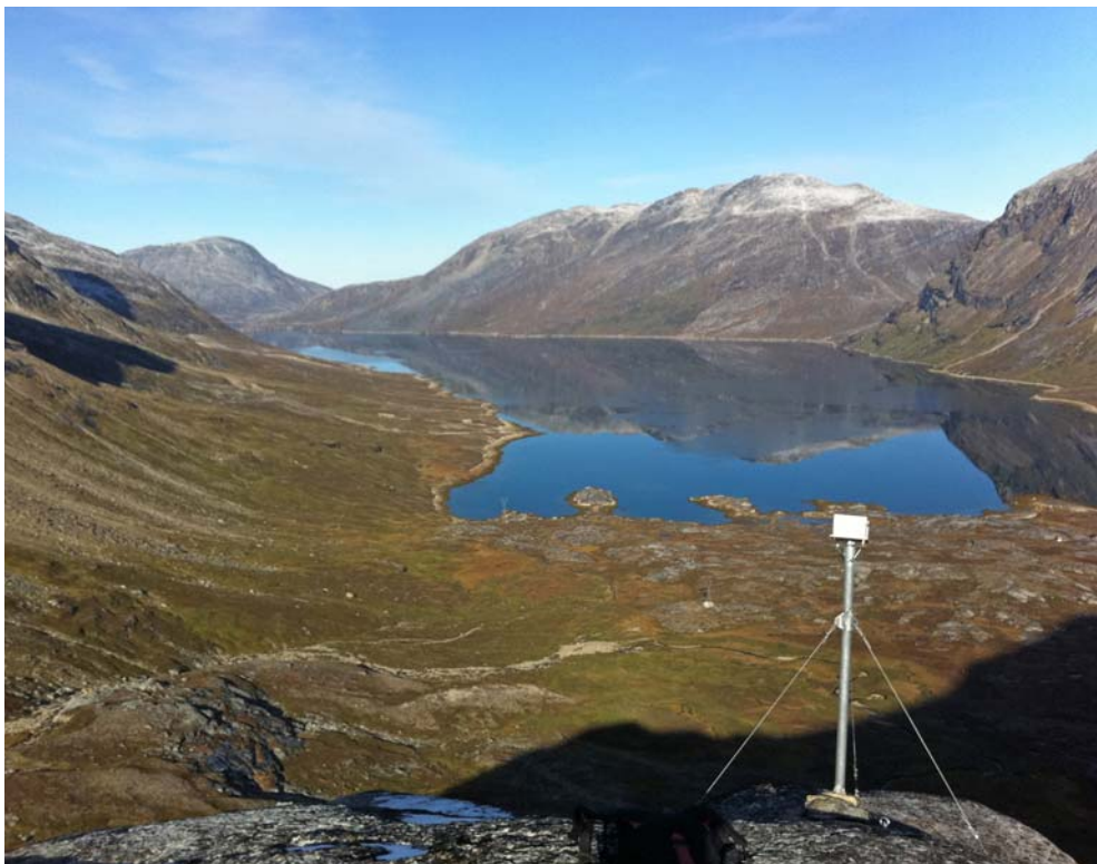
Figure 3.4 Reinstallation of snow camera K1_300 at 300 m a.s.l. (N64o7'26" W51o22'55"). The new camera has been raised approximately 2 m above the terrain to avoid snow formation in front of the camera.
