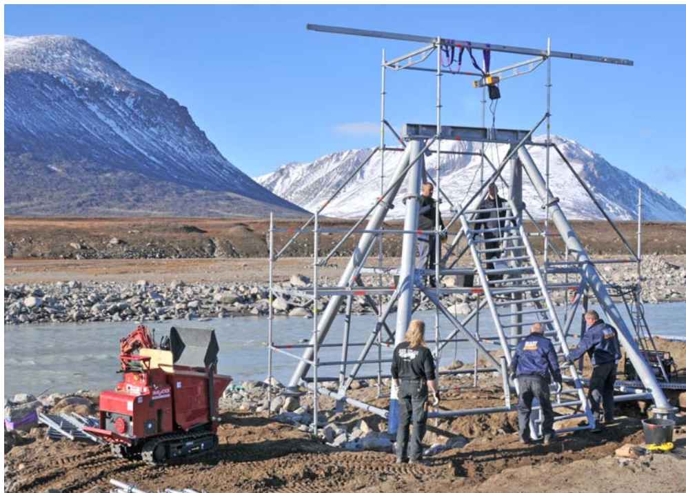
Figure 6.45 The bridge was put together on-site by a crew of seven people using mainly hand power. Photo: Jørgen Skafte.
